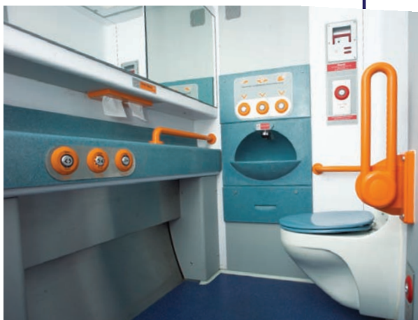
CMEc11 handwasher/driers and vanity units on the South West Trains class 458 carriage.
